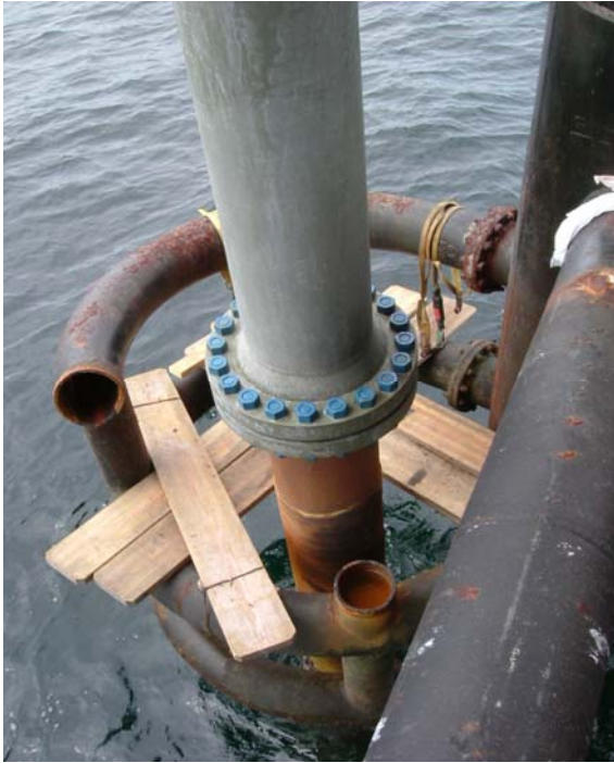
Flange Subject to Splash Zone Corrosion
